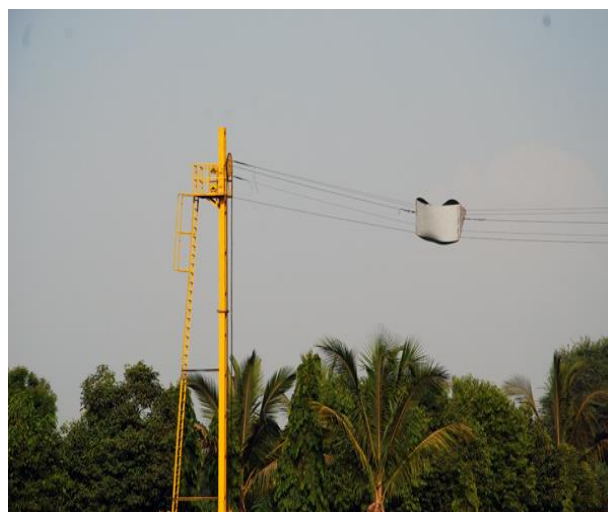
Figure 7: Pole with ladder and platform.
